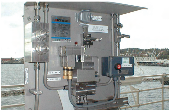
Local Control Panel
