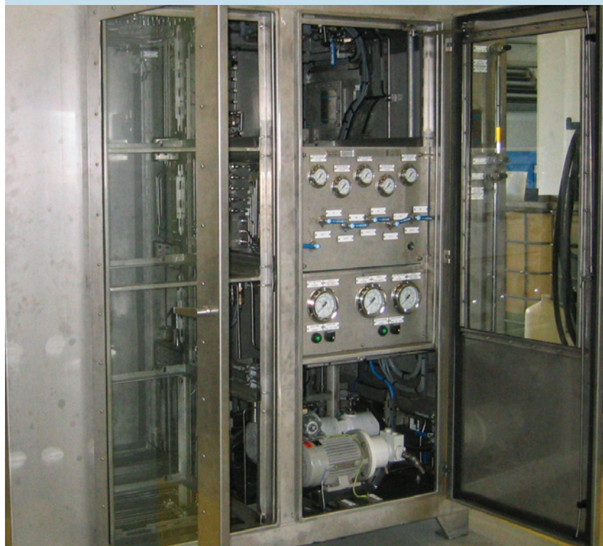
Hydraulic Control System
